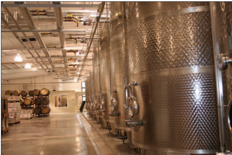
Figure 1. Equipment layout and workflow are critical issues in designing a winery. The winery should have an efficient layout suitable to winemaking and be built to accommodate expansion, when it is needed. (Photo courtesy of Prospero Equipment Corp.)
