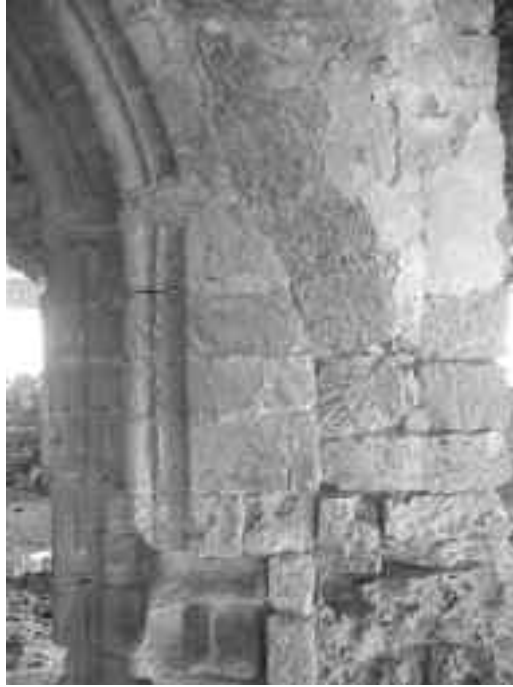
Fig. 5: Piers of the 14 th century dome, showing seam between the original masonry and masonry added in the 16 th century
