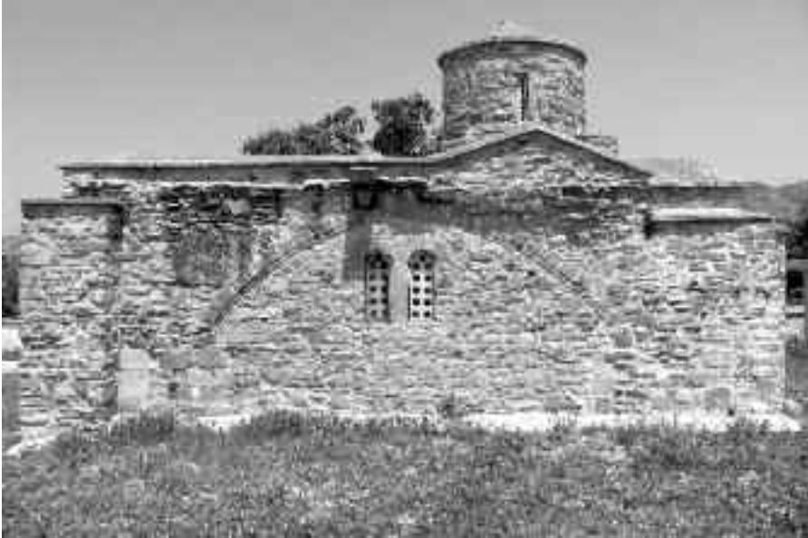
Fig. 15: Profile of early arch in the south side of the church of the Panagia in Kampyli/Hisarköy, Cyprus
