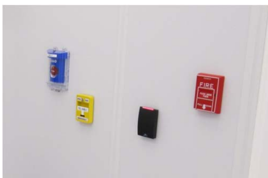
(From left to right) Emergency gas off station (blue), emergency door unlock (yellow), and fire pull station (red).
