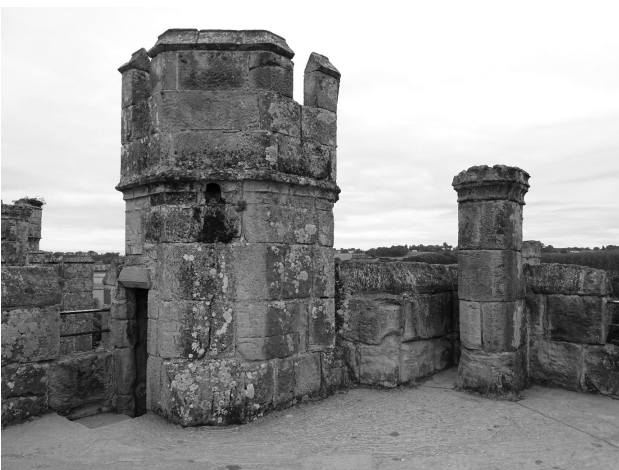
Fig. 3.37: Stair turret and chimney of the north-west tower. Photo by Penny Copeland.
