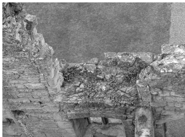
Fig. 3.34: View down only narrow window jamb to west, and rebated door jamb to right. The door jamb sits slightly over the triple door wall at the end of the Great Hall. Photo by Penny Copeland.
