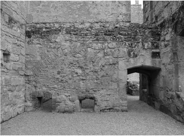
Fig. 3.15: Southern cross wall of western range showing relieving arch and flue or stoke holes. A further retaining arch is visible on the northern side. Note knife sharpening effect on doorway. Photo by Penny Copeland.
