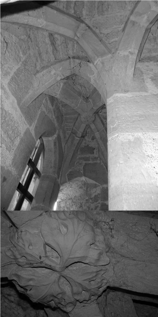
Fig. 3.17: Leafy boss in the first floor corridor of the gatehouse. Photos by Penny Copeland.
