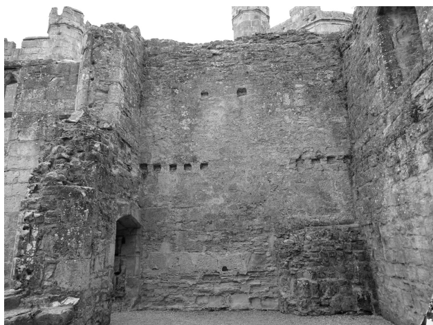
Fig. 3.38: Floor joists with gap for trimmer and faint scar in surviving plaster for staircase from ground floor against the external northern wall of the kitchen. Note the rebuilt oven below. Photo by Penny Copeland.
