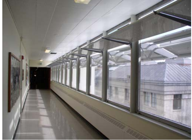
Fig. 2: Light shelf inside the hallway reflects light to the ceiling and spreads the daylight further into the building. LED lighting can be seen on the outer edge of the light shelf. Florescent lighting on the ceiling will be removed when the LED lighting becomes operational.
