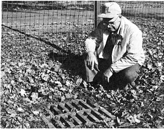
A protective grate on a surface inlet
