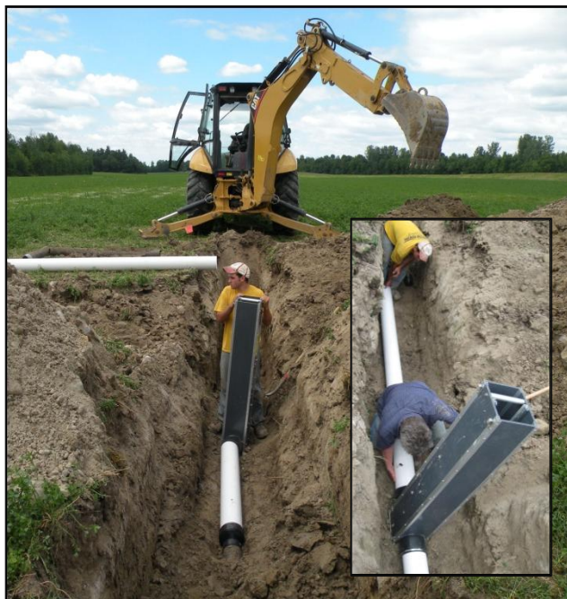
Figure 2: Installation of a water control structure in a field at the Miner Institute.
