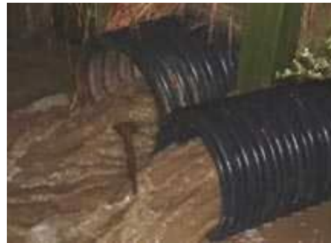
Regular observation and monitoring of subsurface drains is required to prevent surface contamination of liquid animal wastes. Photo courtesy of Jon Rausch, OSU Extension
