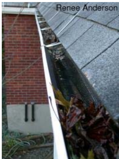
A clogged rain gutter on a house provides the conditions for mosquito larvae to develop.
